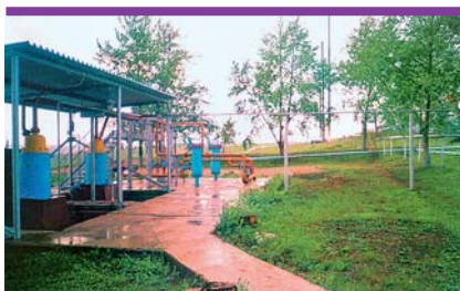
Yakeevskaya pump station for transportation of natural gas liquids equipped with tight electric pumps GEN 50/400 (JSC Tatneft)
