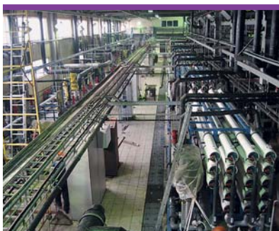
Tatneft petrochemical plants, JSC Taneko: Water treatment for fine desalination of water, capacity 1,000 m 3 /h
