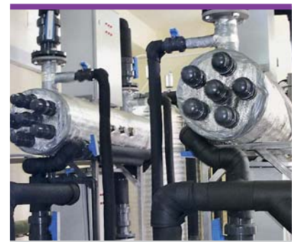
OJSC Nizhnekamskneftekhim: Purification system for oil containing condensates, capacity 800 m 3 /h, TOC \leq 200 \mu\text{g}/\text{dm}^3
