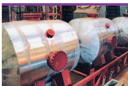
Steam separation unit for Verkhne-Mutnovskaya Geothermal Power Plant
