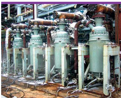
Pump station of AVT-5 unit (gasoline production) equipped with tight electric pumps GEN 170/190 and GEN 90/100 (JSC LUKOIL-Nizhegorodnefteorgsintez)
