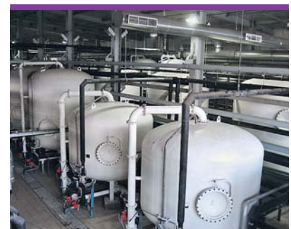
JSC Sibur-Khimprom: Water treatment for desalination, capacity 700 m 3 /h, \text{æ} \leq 0.2 \mu\text{S}
